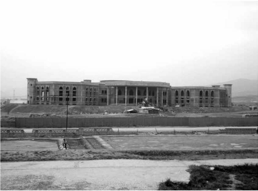
The new Parliament Building in Afghanistan is being constructed by Government of India
